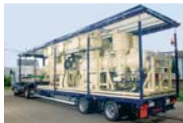
This 4-bays mobile substation is intended to power the distribution grid in case of emergency.
