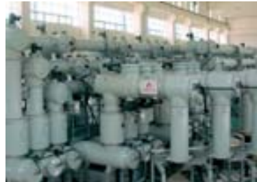
This 500 kV GIS feeds a transmission system with power generated by a hydraulic power plant.
