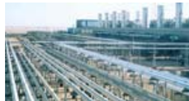
420 kV GIL: 17 km in a thermal power plant.
