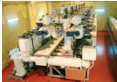
B105 GIS 245 kV in a city center.
